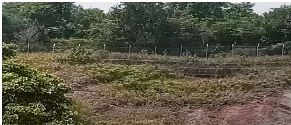
Diagram 1.4 (a): New Fence Installed in Front of the Immigration, Customs, Quarantine & Security Complex - ICQS Biawak
